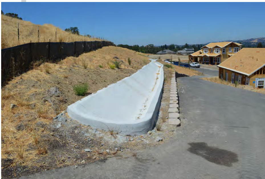
The GHAD has full responsibility for the concrete v-ditch used to collect storm drainage.
