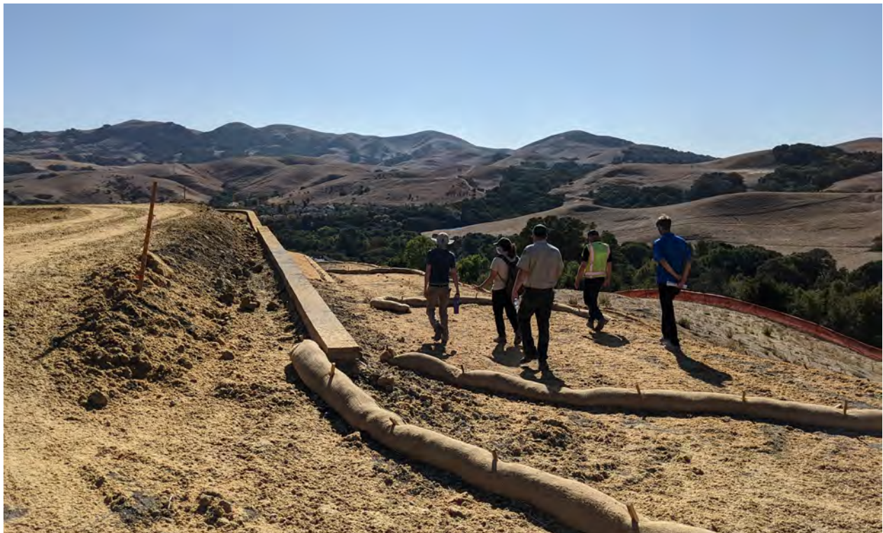
The Saudade Walk-in Entrance from the Faria Preserve HOA area will connect trail users to the Calaveras Ridge Trail (seen under construction in the photo above).
